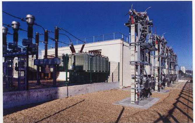
The Deschamps sub-station
