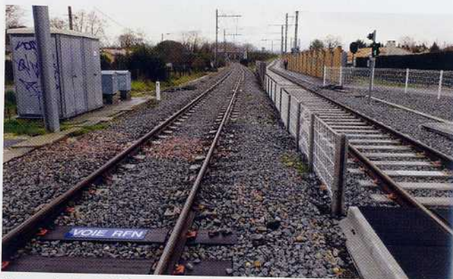
Towards the Médoc area : two adjoining infrastructures. Management of level crossings and other consequences
